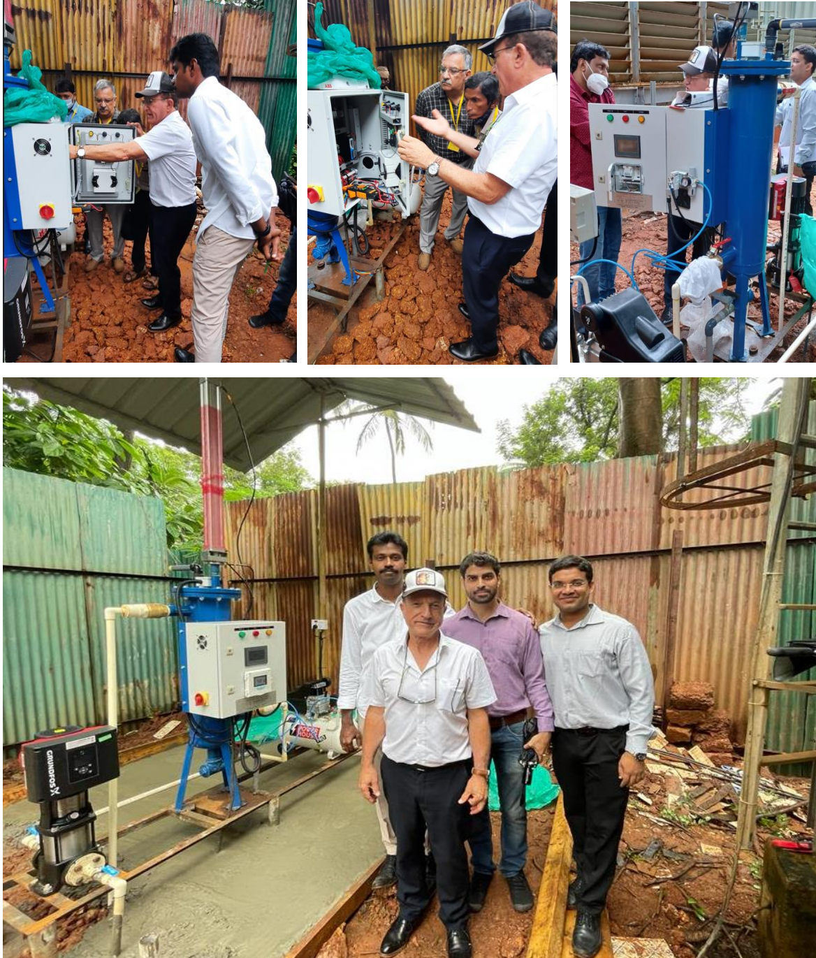
Figure 7: Commissioning photos of EST system
