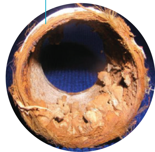
Corroded pipe with treatment
