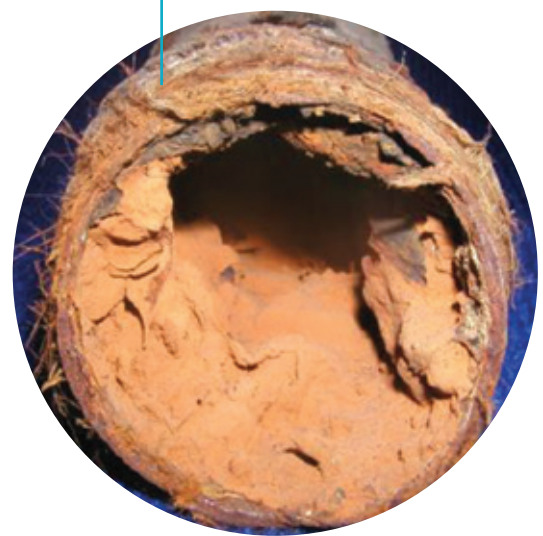
Corroded pipe without treatment
